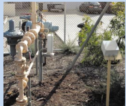
An installation of the DL220 at an industrial meter station
